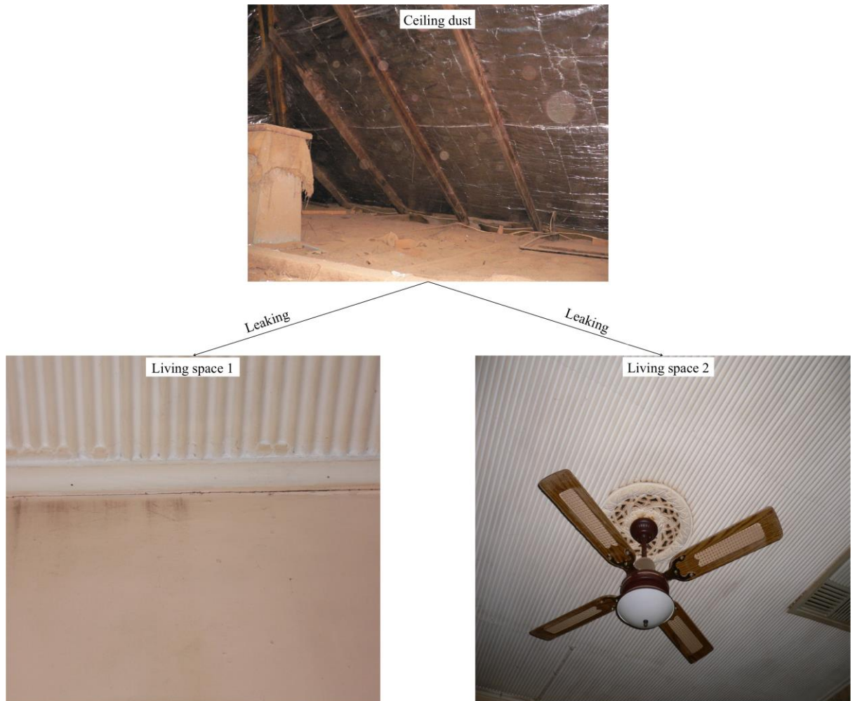
Supplementary Figure S6. Contaminated ceiling dust leaking into living spaces in older Broken Hill homes.
