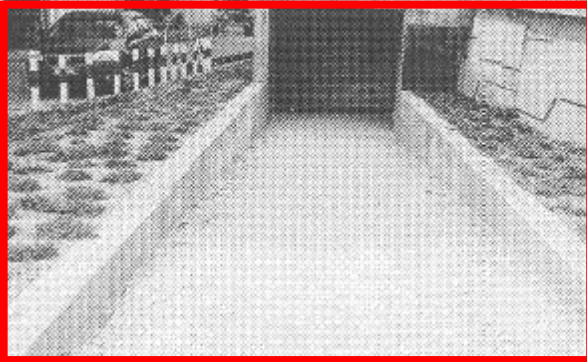
No help: The path that leads to the underpass does not have railings to support the disabled.
